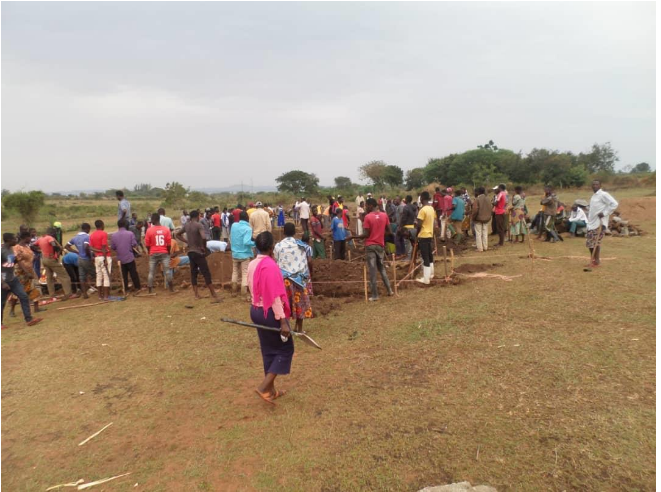
Community members mobilized to participate excavation of foundation trench for constructing their HCF, Kyamwame village
